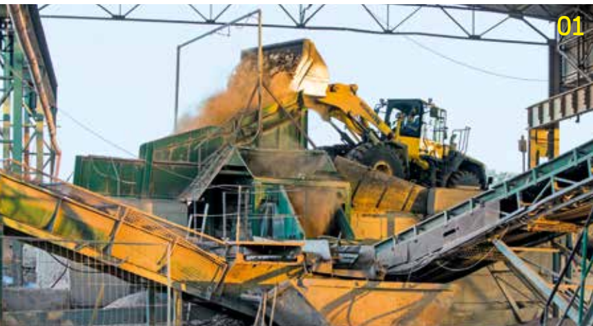
01 Recycling Centre Himberg, Himberg
